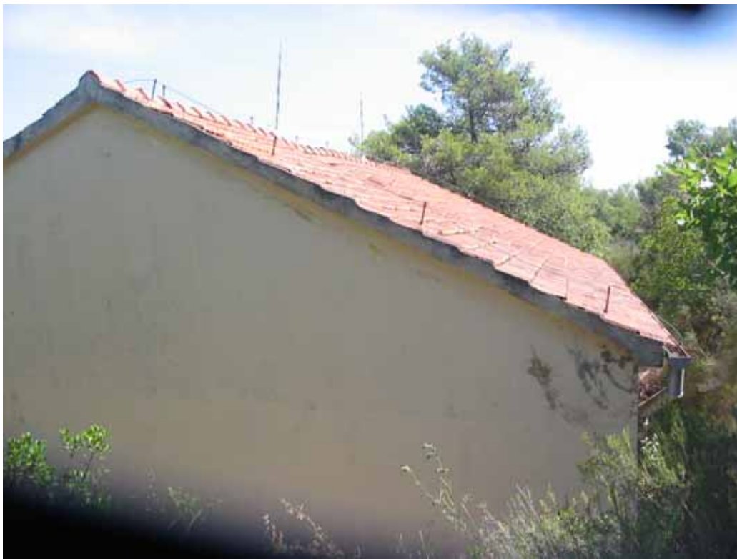
Photo nr.4. View on the south side of the roof and the west wall
